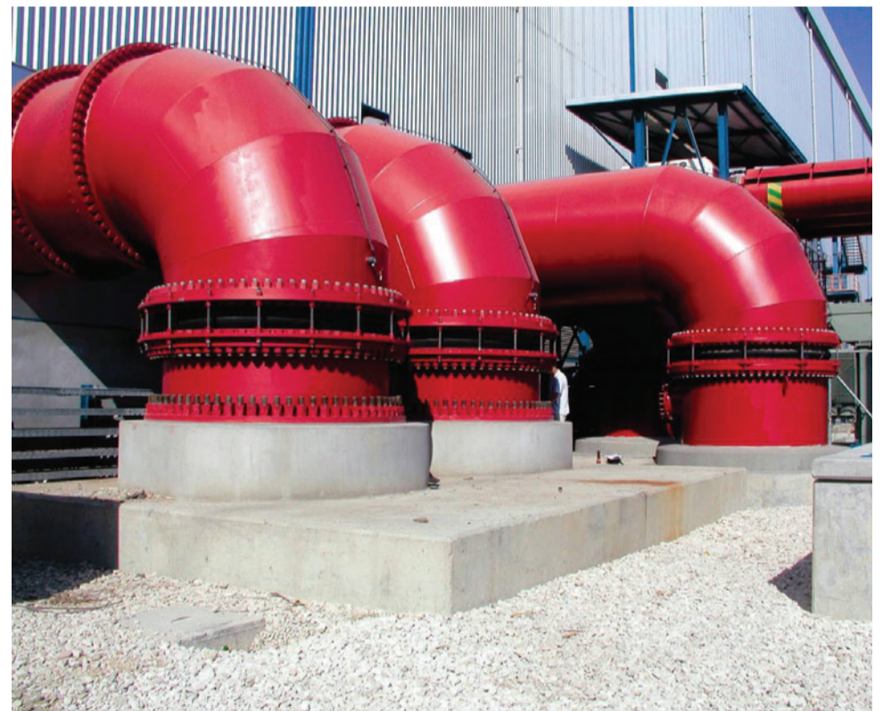
Rubber cord expansion joints on the pipeline
